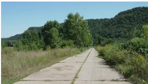
18 foot wide concrete pavement south of Weaver (Wabasha County) – part of State Route 3, one year before marked as US 61
