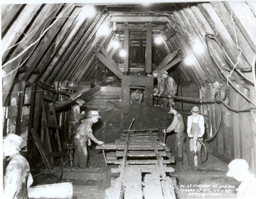
Seven workers are shown in the tunnel being constructed in the stream sediments of Glacial River Warren terrace east of downtown St Paul. At this location, about 112' below Lafayette Rd and Grove St, a 13'-3" semi-elliptical section of the Joint Interceptor sewer was constructed in 1935.
