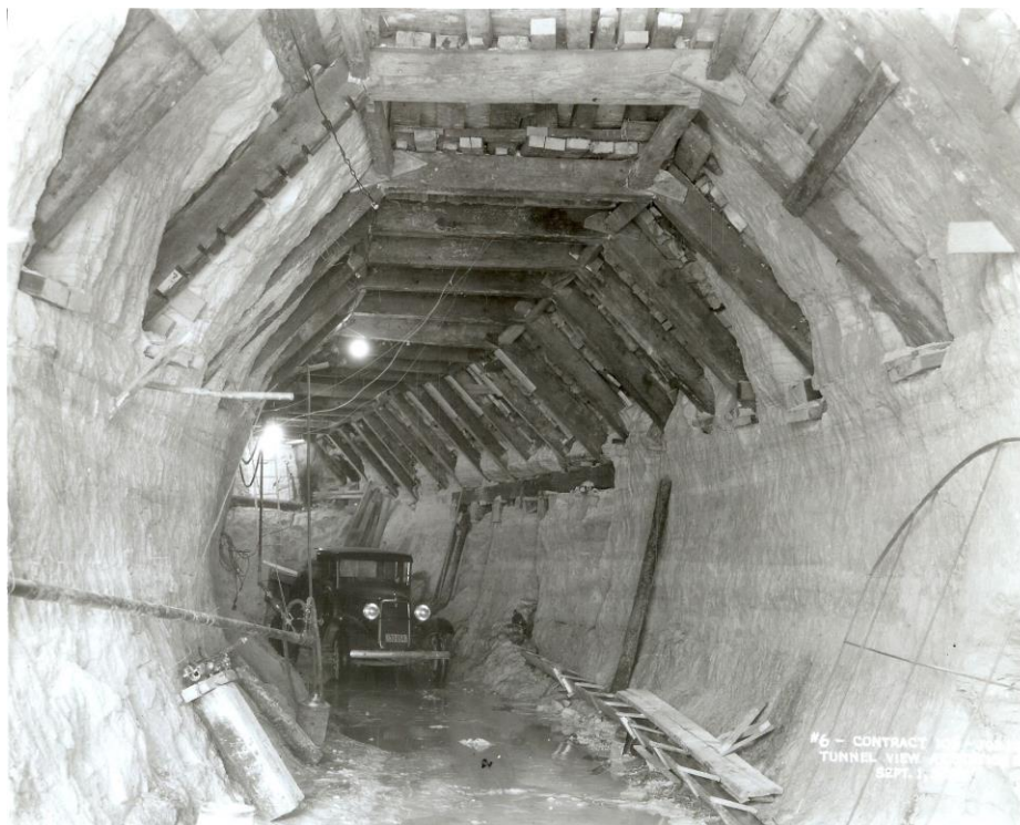
The furthest downstream tunnel constructed in the St Peter Sandstone exited St Paul's Dayton's Bluff north of Warner Rd east of its intersection with Childs Rd, which allowed entry of the vehicle. The Joint Interceptor section here is a 13'-10" circular sewer completed in 1935. About 1200' upstream from the location of this photo the sewer invert is 212' below the surface.
